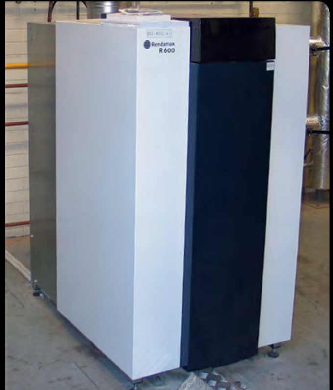
New gas fired condensing boiler
