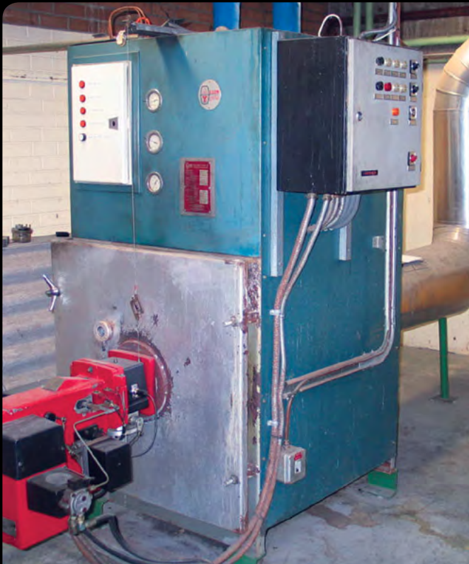
Old 1970s gas fired heating boiler
